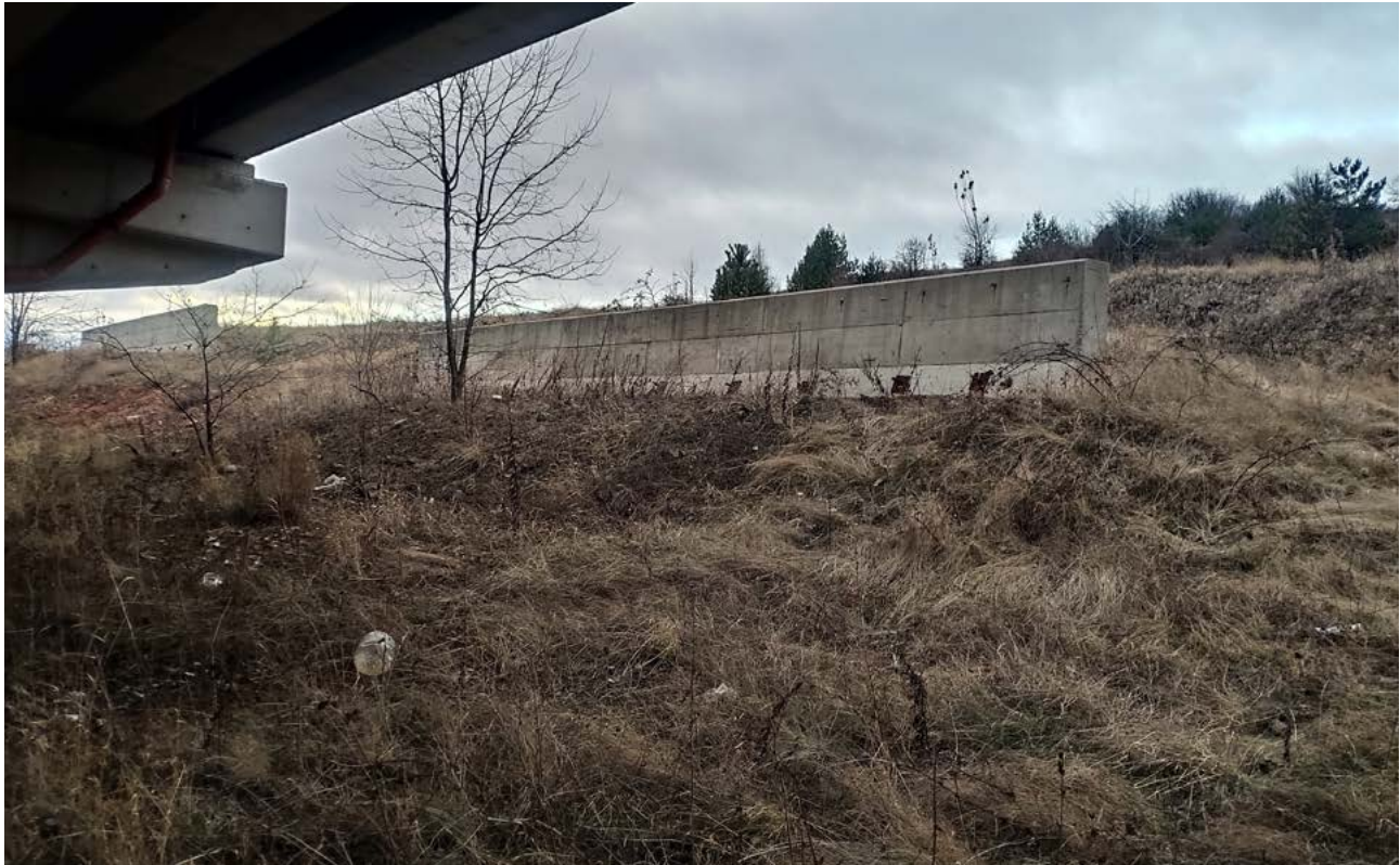
Fig 12. Concrete wall blocks 50% of the northern site of the viaduct of Struma Motorway Section 1 (© BBF).
