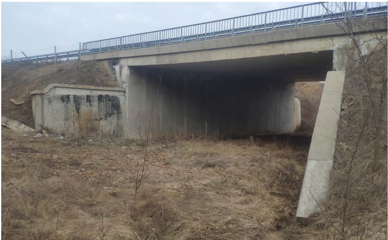
Fig 13. An underpass for wolves at Struma Section at 1 km 315+900, 42°21'42.37" 23° 6'14.60" Concrete wall blocks 50% of the northern site of the viaduct of Struma Motorway Section 1 (© BBF).
