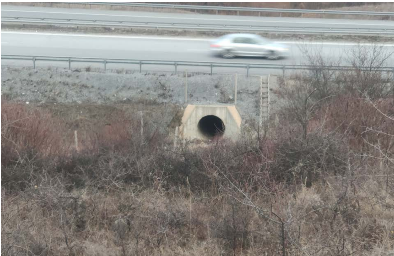
Fig 17. Other existing wildlife crossing facilities at Struma Motorway Section 1 that serve or could serve as defragmentation facilities (© BBF).
