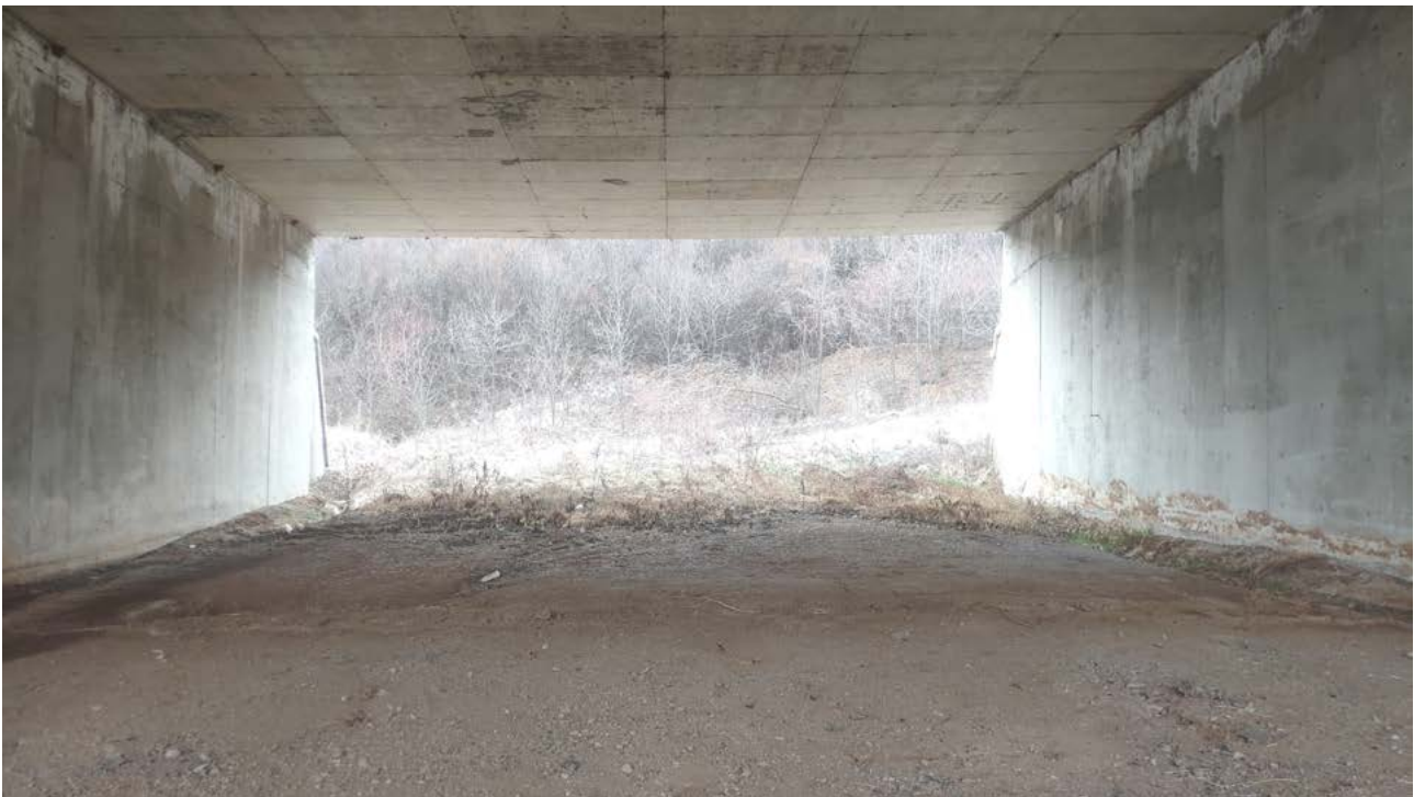
Fig 14. A bare surface in the underpass for wolves at Struma Section at 1 km 315+900, 42°21'42.37" 23° 6'14.60" (© BBF).
