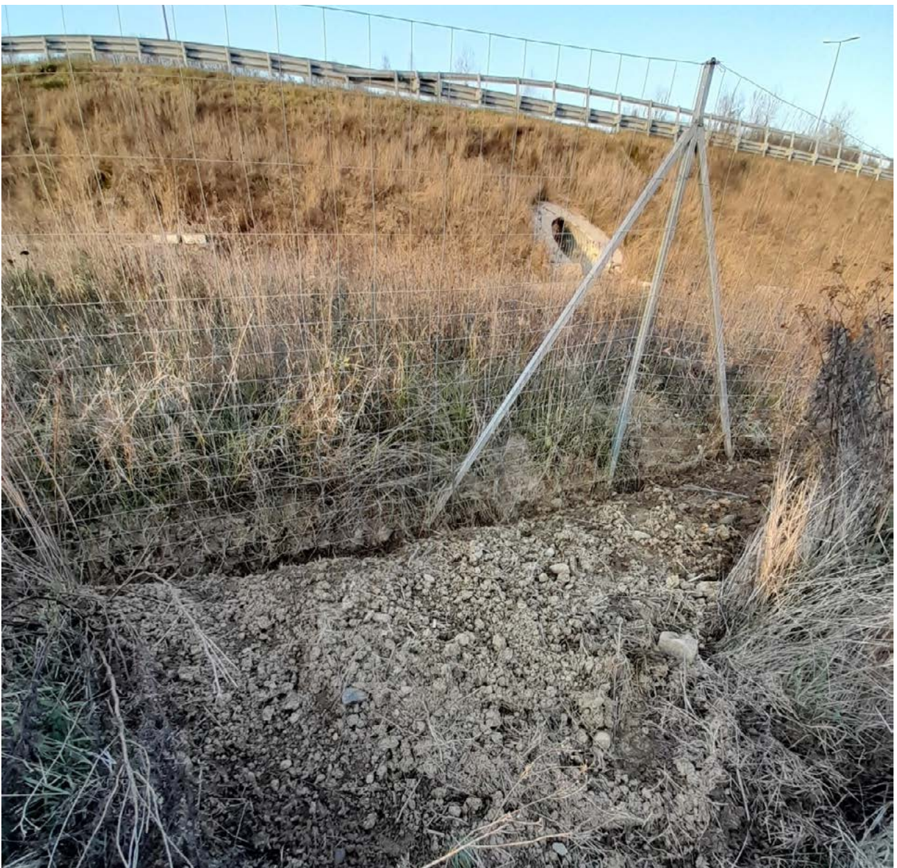
Figure 5 A culvert not yet integrated in the surrounding terrain (upper left); a culvert interrupting the water connectivity during a drought period (upper right); a culvert blocked by the fence of the motorway with badger diggings under the fence (bottom). (© Zarand)
