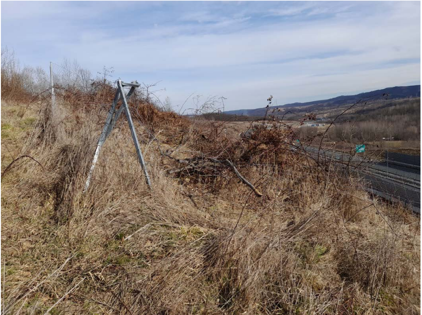
Figure 17 Existing fence is not bear-proof and is not being maintained regularly (© Zarand)
