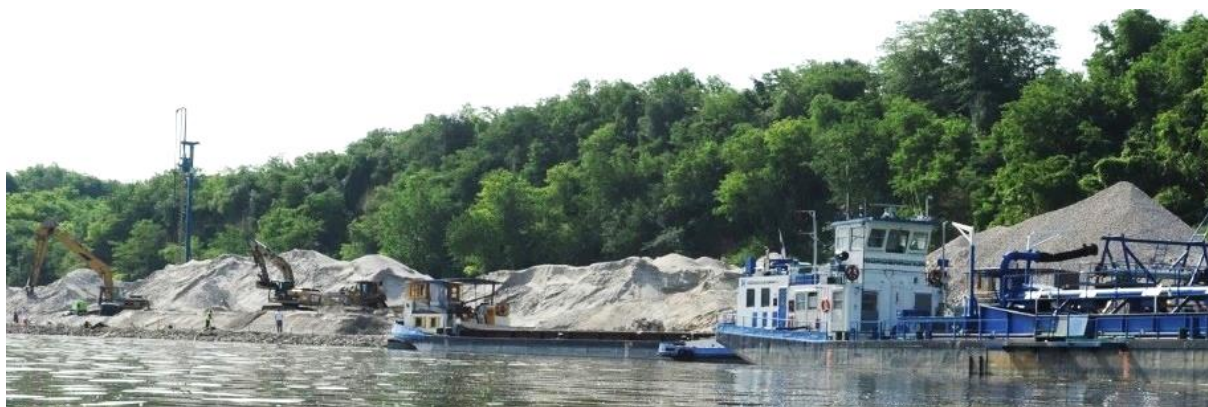
Figure 5&6: Bank reinforcement on the Danube near Vukovar, Images: WWF/Arno Mohl, Darko Grlica.
