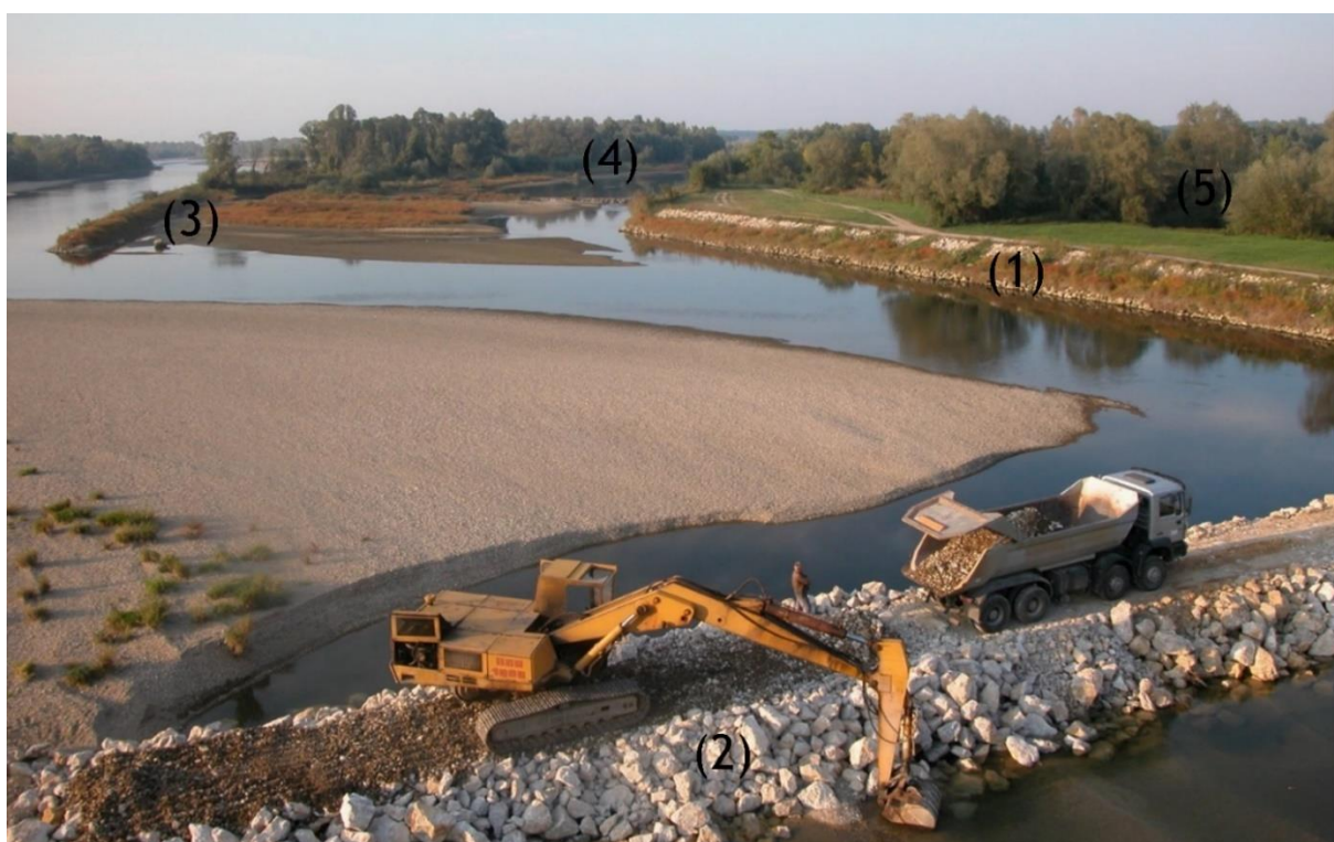
Figure 7: The typical repertoire of river regulation in the project area: Groyne construction in the foreground (2), bank protection on the right side (1), training wall on the left upper side (3) and cross dyke (transversal fill) closing the side channel in the upper central part (4). Finally, the flood dyke (5), immediately behind the softwood (invisible), complement the regulation works. © Credit: WWF/ A. Mohl.
