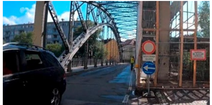
Figure 16: Problematic traffic signs at construction site, with not safe detour route at EuroVelo 14 in Austria
