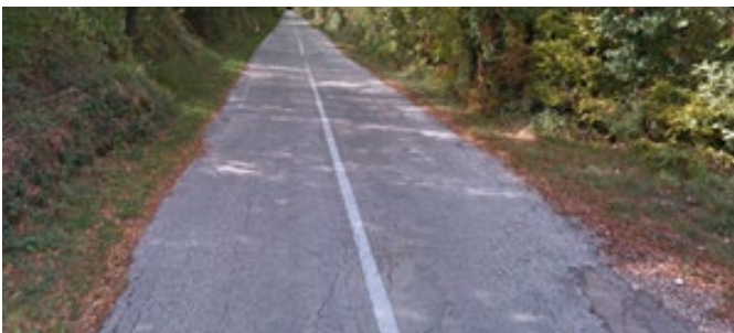
Figure 13: Potholes and damage due to tree roots at EuroVelo 8 in Croatia
