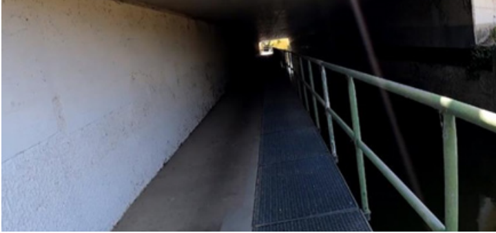
Too narrow bicycle infrastructure at an underpass on the EuroVelo 9 in Austria [11]
