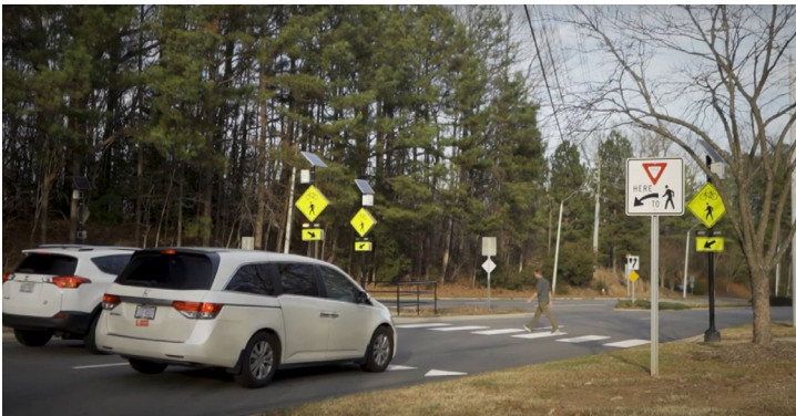
Rectangular rapid-flashing beacon installed on a pedestrian crossing, USA [6].
