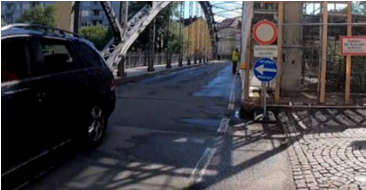
Problematic traffic signs at construction site, with unsafe detour route at EuroVelo 14 in Austria [10]
