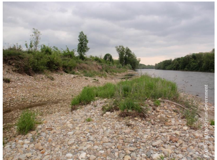
Bank erosion at the main channel of Mura river, May 2010
