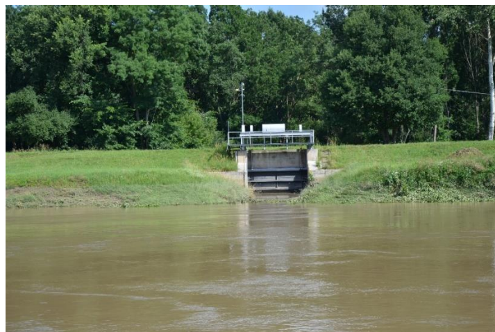
Figure 27: Inflow object to the retention area behind the flood protection dyke (Author: VUVH)
