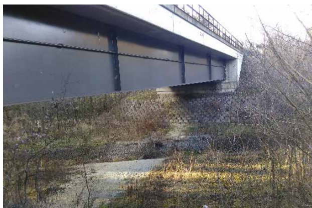
Figure 32a and b. Location and image of the railway bridge. Photo: Danial Mach, https://www.szdc.cz/stavby-zakazky/prehled-projektu/-/projekt/detail/54970973
