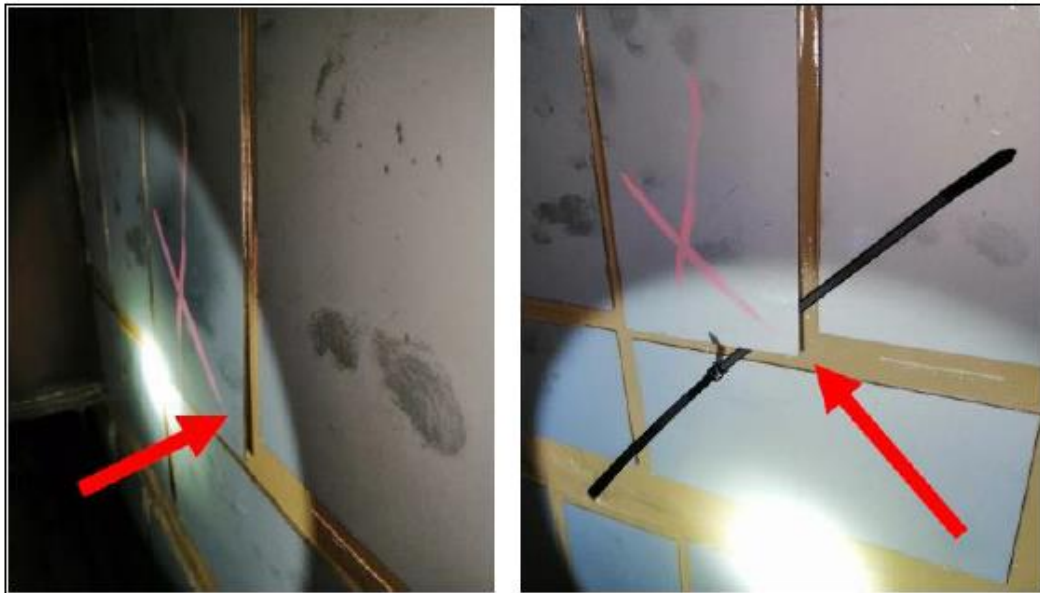
Abstract from developed technical report after survey performed on board, check of damping treatment correct application
