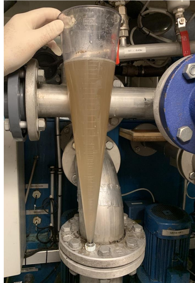
Reject water to river
