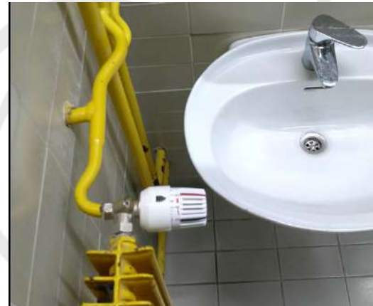
Thermostatic valve in the toilets
