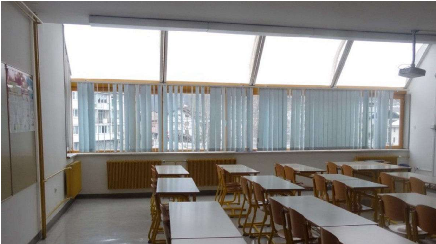
Unconventional pipelining installation – Four radiators in the room are supplied from three different sources
