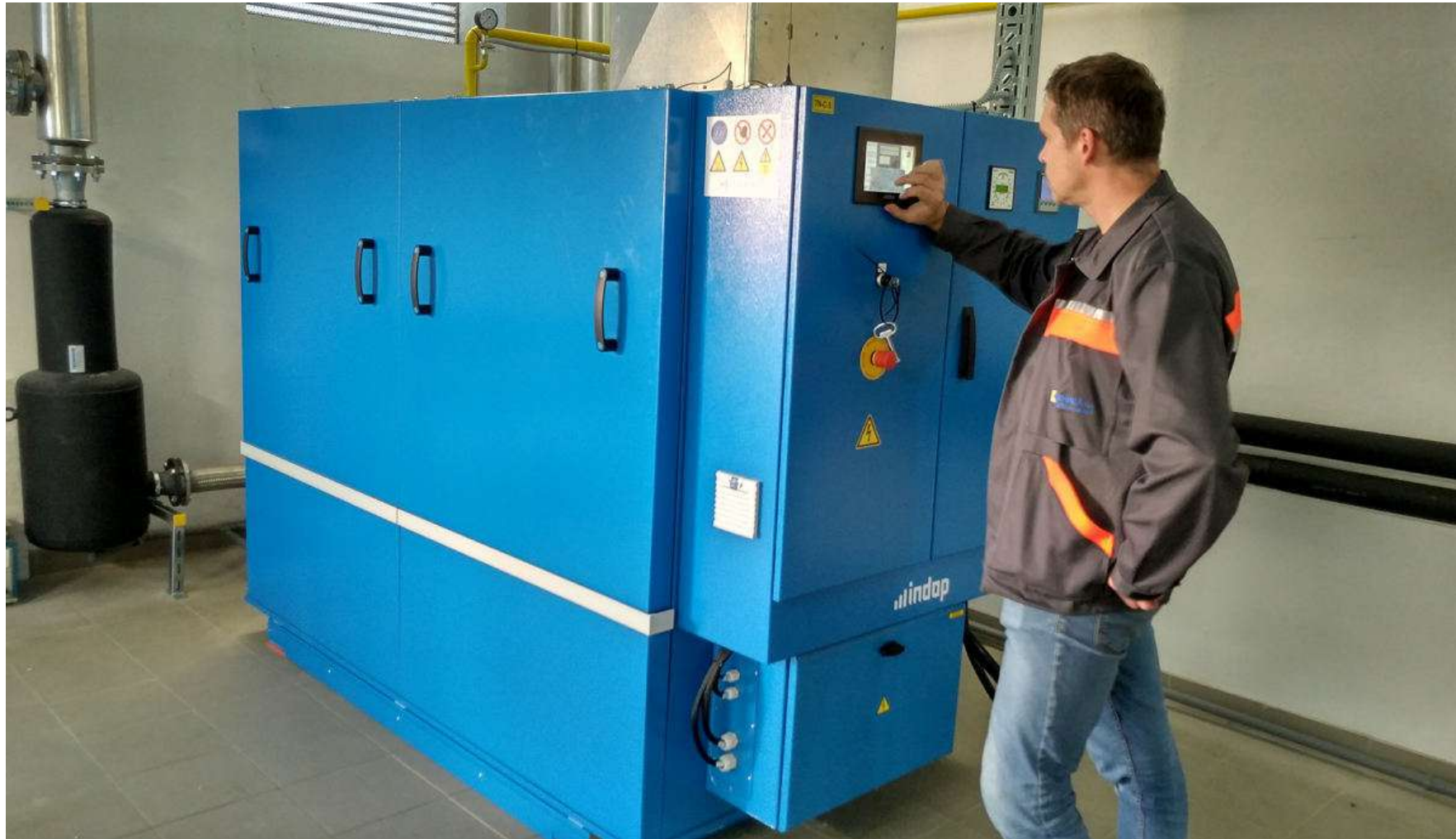
CHP unit in boiler room
