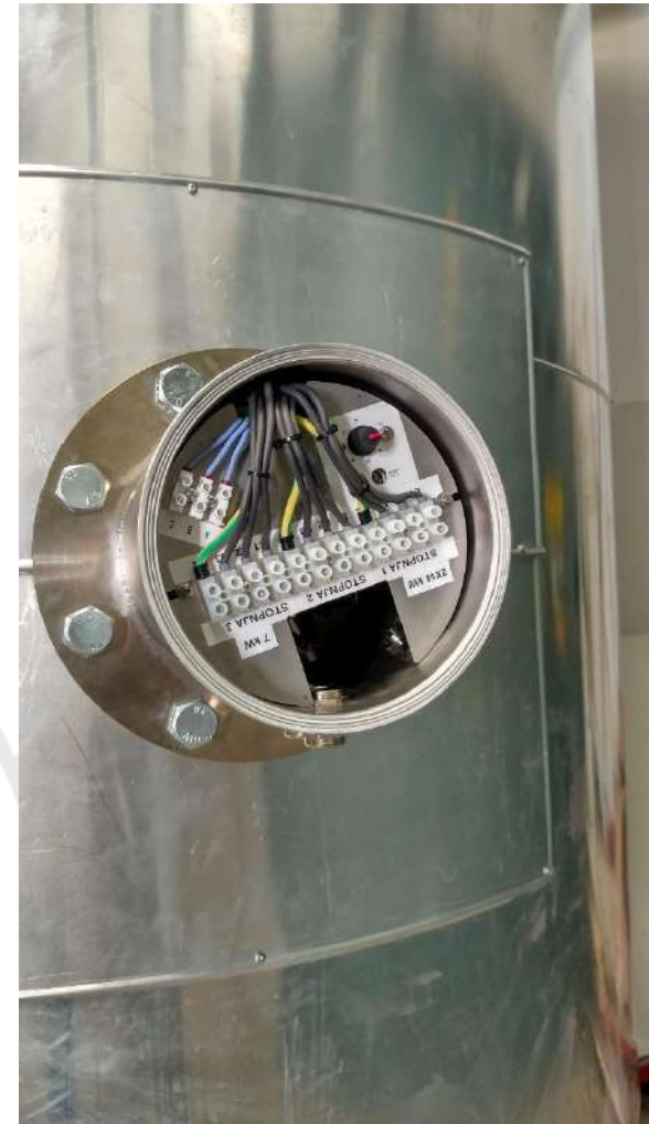
Electrical heaters, 35 kW
