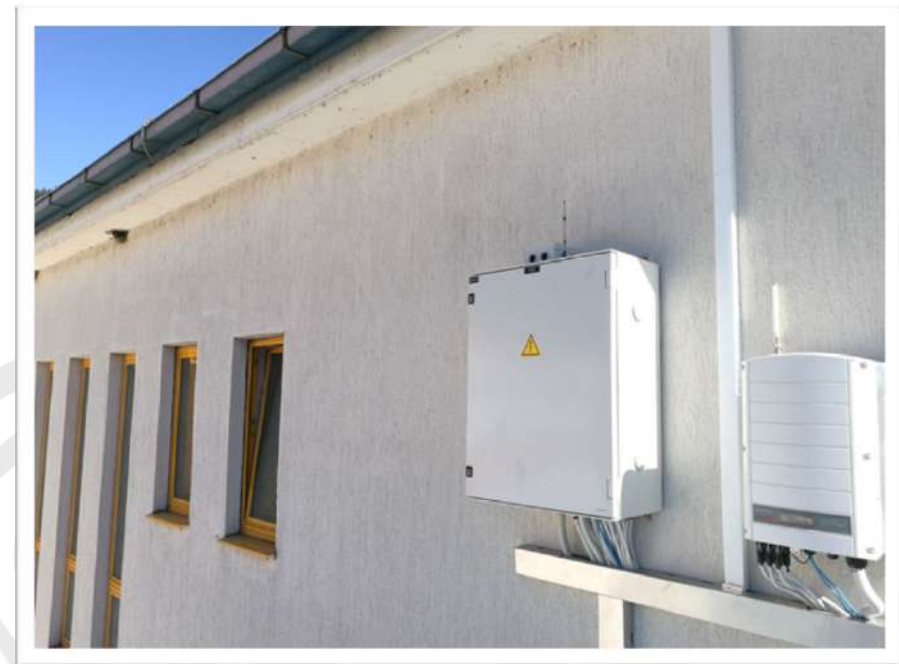
Electrical installations cabinet and inverter box
