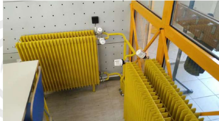
Attempt to resolve underfed radiators in distant locations with adding more radiators
