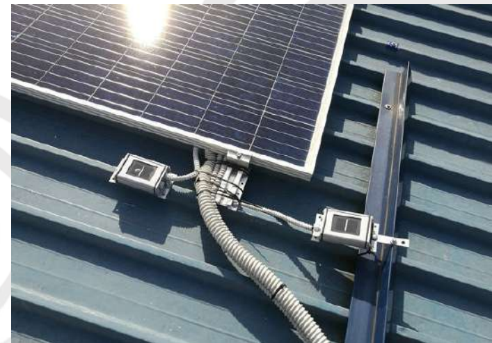
Solar irradiance sensor
