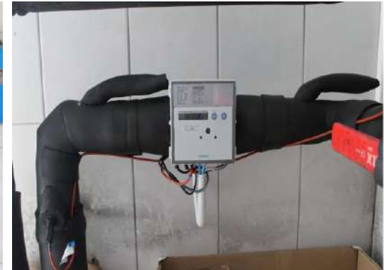
Calorimeter for heat pump Siemens UH50-C60-BA06-E
