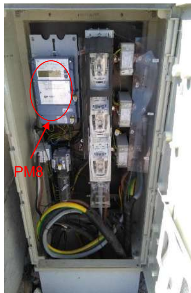
Electric meter Sentron PAC 2200 for battery system
