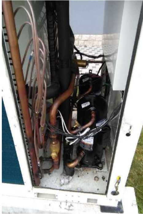
New compressors Copeland ZP182 for heat pump
