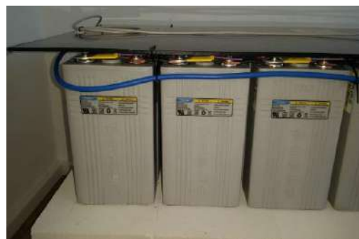
Battery cells with battery management system
