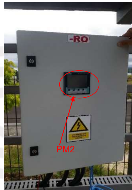
Electric meter Sentron PAC 3200 for PV plant
