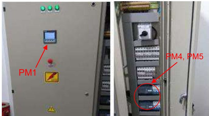
Electric meter at the building's main electrical cabinet Siemens SENTRON PAC3200 and Siemens SENTRON PAC2200
