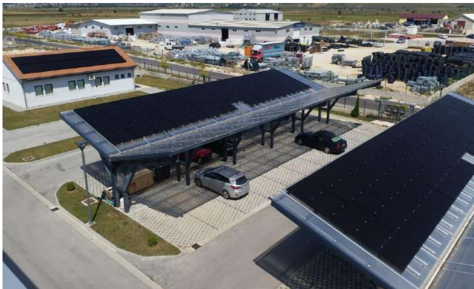
PV panels, 166 pcs
