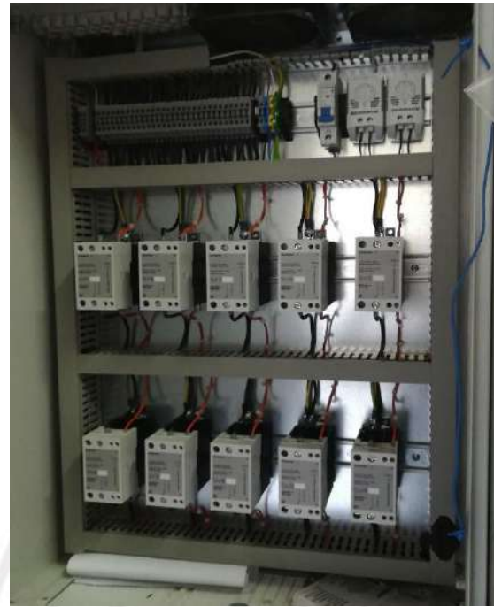
Electrical cabinet RO-EOTB for electrical boiler automation with SEA45.1 current valves and SEM62.2 transformer
