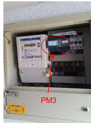
Electric meter Sentron PAC 2200 for battery system
