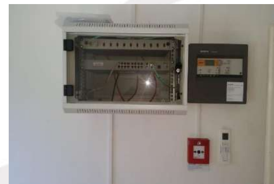
Communication rack, autonomous fire alarm device
