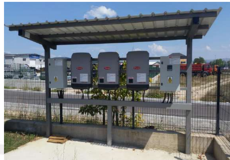
DC/AC inverters, AC and DC electrical cabinet
