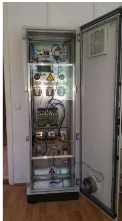
Power converter rack, two-way AC / DC converter Cognito type Open4Lab
