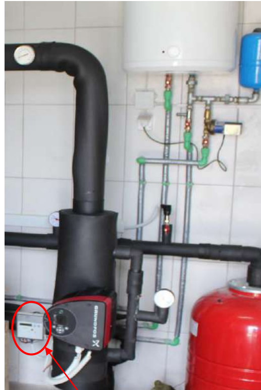
Central calorimeter for measurement of entire heating/cooling energy towards FCU, Siemens UH50-C60-BA06-E
