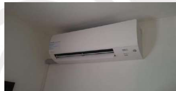
Air conditioning unit: Daikin RX50/FTX50
