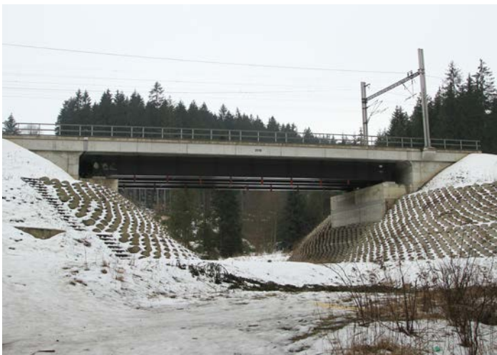
Fig. 57: Underpass constructed on the railway in the Mosty u Jablunkova cadastre close to national border (photo by Ivo Dostál / Transport Research Centre).
