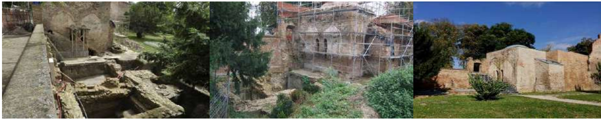
Works on the reconstruction of the hammam afeter researches, 2013; Hrvatski restauratorski zavod
