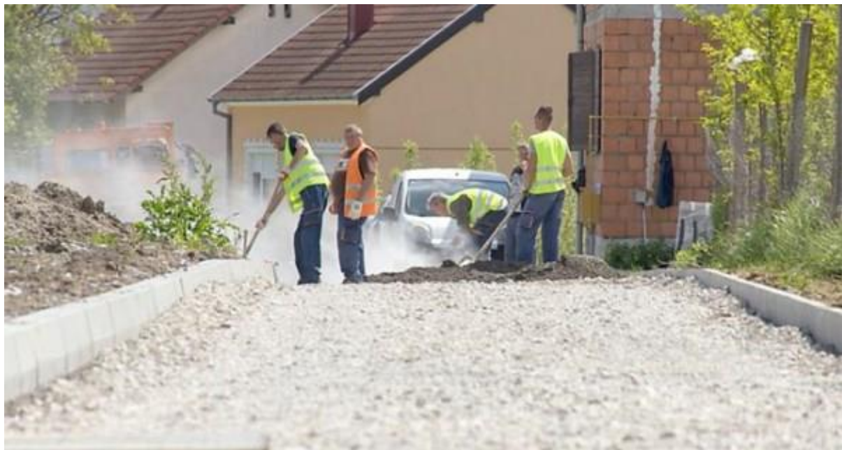
Figure 23: Construction of the bike path in Vukovar-Borovo route Source: City of Vukovar image database
