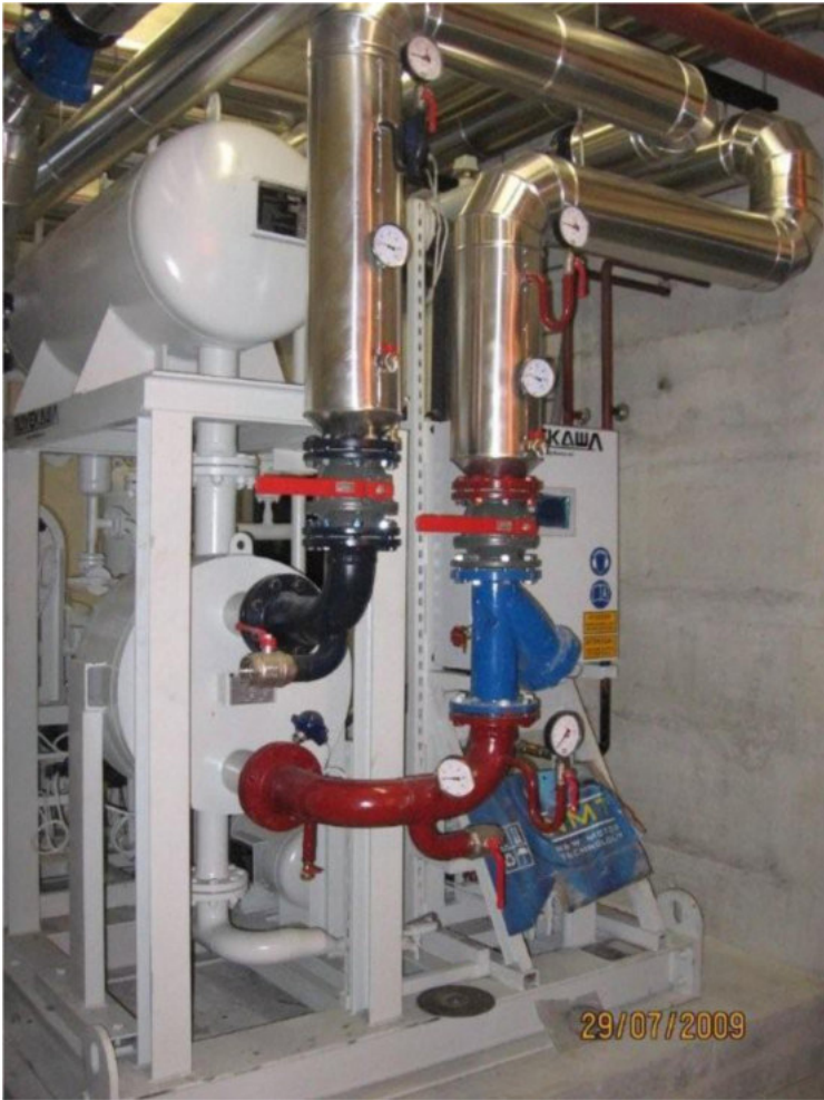
Figure 21: Installed high temperature heat pump
