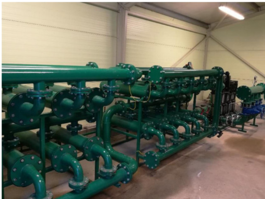
Figure 20: 20 in 10 \mu m filters in engine house near the (re)injection well
