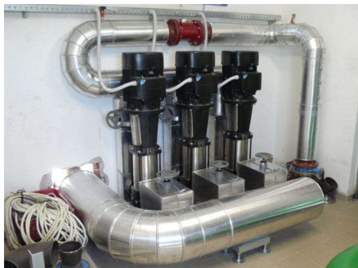
Figure 1: Installed group of booster pumps
