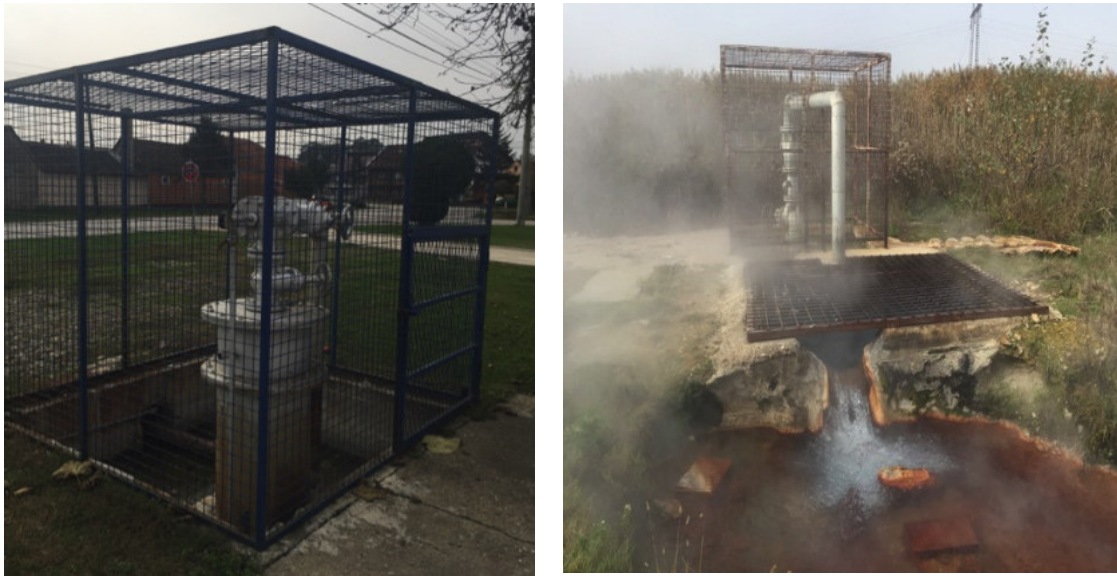
Fig. 30: Hydrogeothermal well BB-1, Bogatić (on the left) BB-2, Bogatić (on the right)
