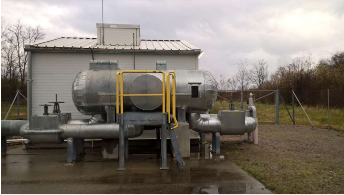
Fig 18: The reinjection well (K-23) with mechanical equipment
