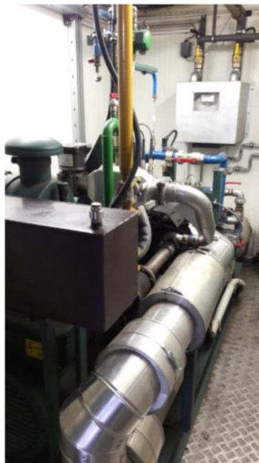
Fig. 27: The 50 KW gas engine CHP plant
