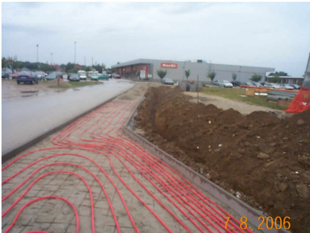
Fig. 39: Lendava de-icing: De-icing of pavements in Lendava as a part of a district heating system with geothermal energy
