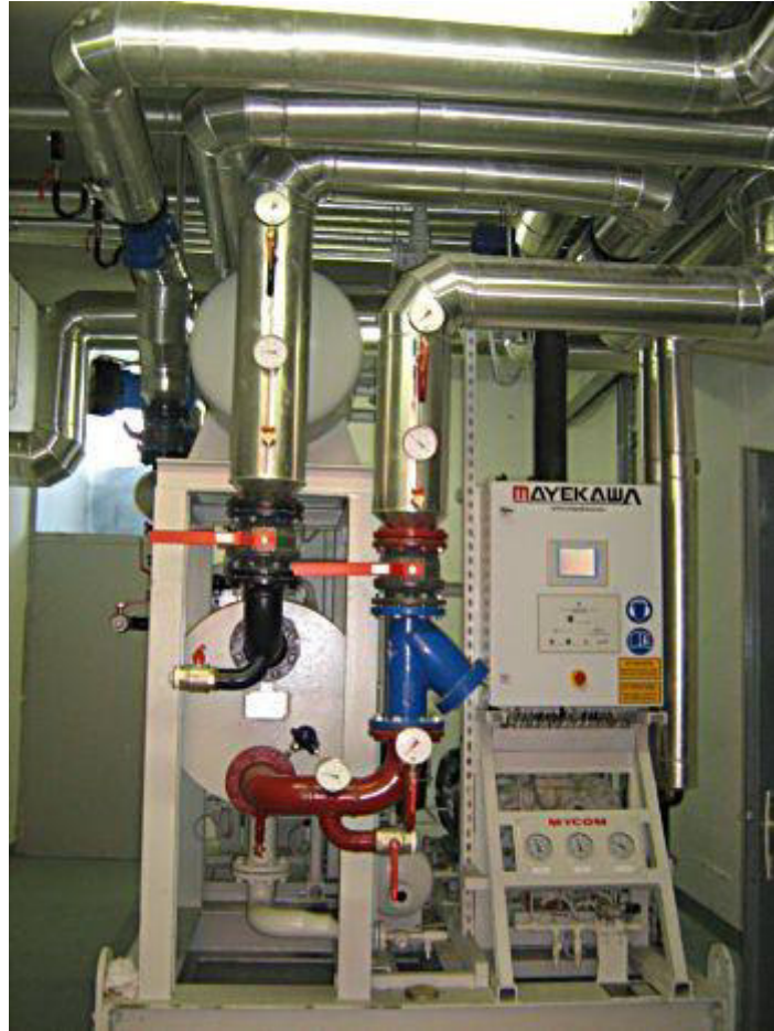
Fig. 37: High emperature heat pump in the Lendava district heating system (Petrol Geoterm website).
