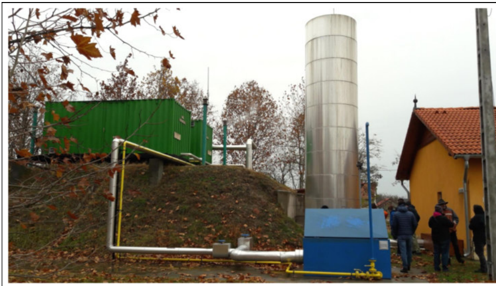
Fig. 26 The production well (B-45) and the gas separator in the Hunyadi Park, Mórahalom
