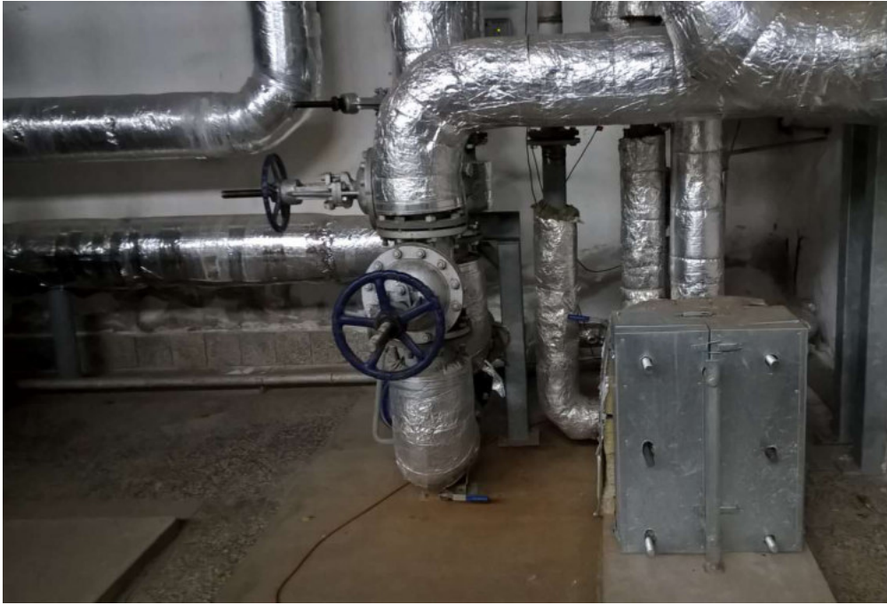
Fig. 16: The heat exchanger with mechanical equipment
