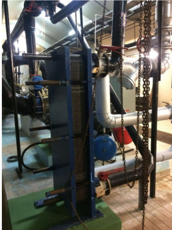
Fig. 10: Heat exchanger inside the complex of SRC-a Mladost (photo: D. Šolaja).
