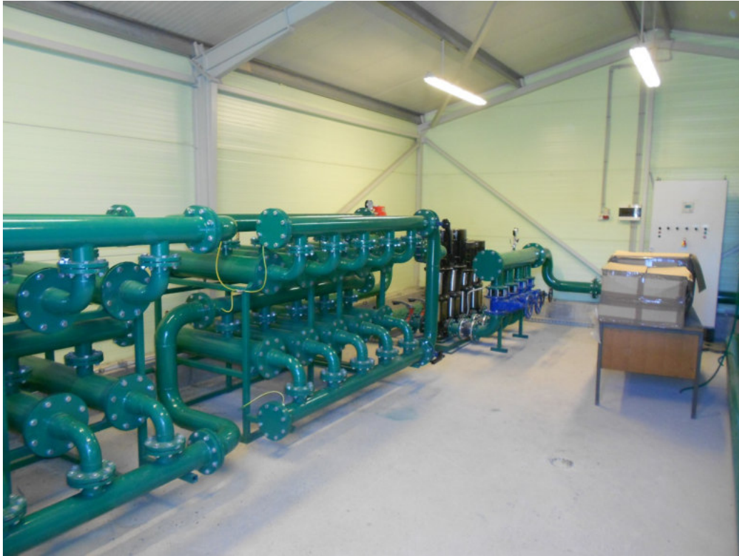
Fig.38: Nafta Geoterm object - fibre filters for waste thermal water before being reinjected into Le-3g well in Lendava
