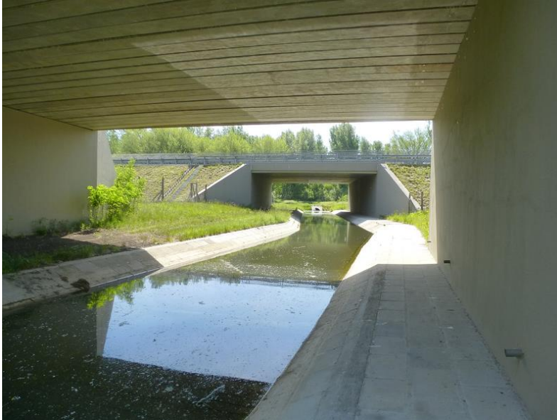
Barbacs-channel in crossing zone of M85 and m.r.85 Bad concept and desing: lost of several ecological function and high number of road kill of mammals
