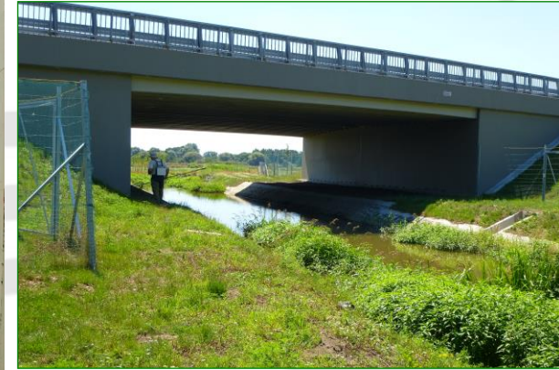
Keszeg ditch in the crossing zone of M86. Ecological corridor for aquatic and terrestrial species.
