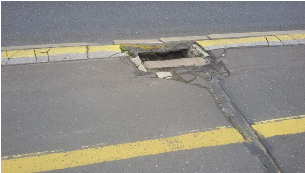
Figure 128. Unmaintained and dangerous gully grate on the cycle track. Source: Sindikat biciklista
