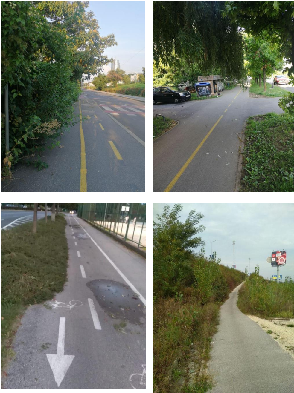
Figure 129. Poor vegetation maintenance. Source: Sindikat biciklista
