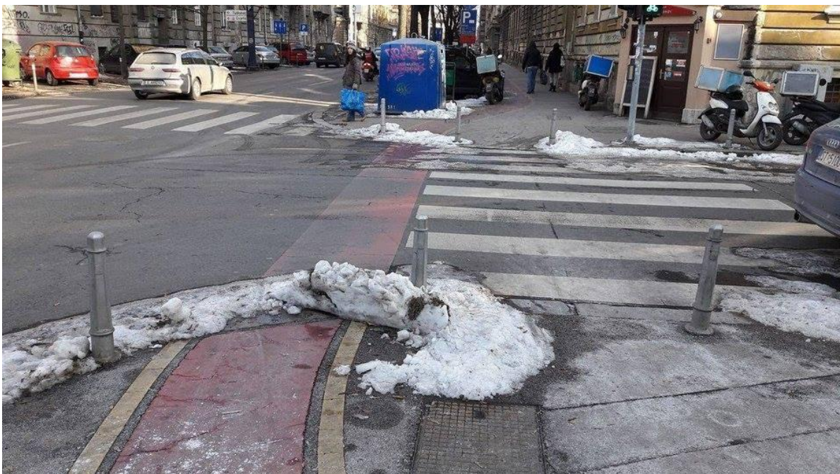
Figure 132. Example of poorly maintained cycling infrastructure in winter conditions. Source: Sindikat biciklista
