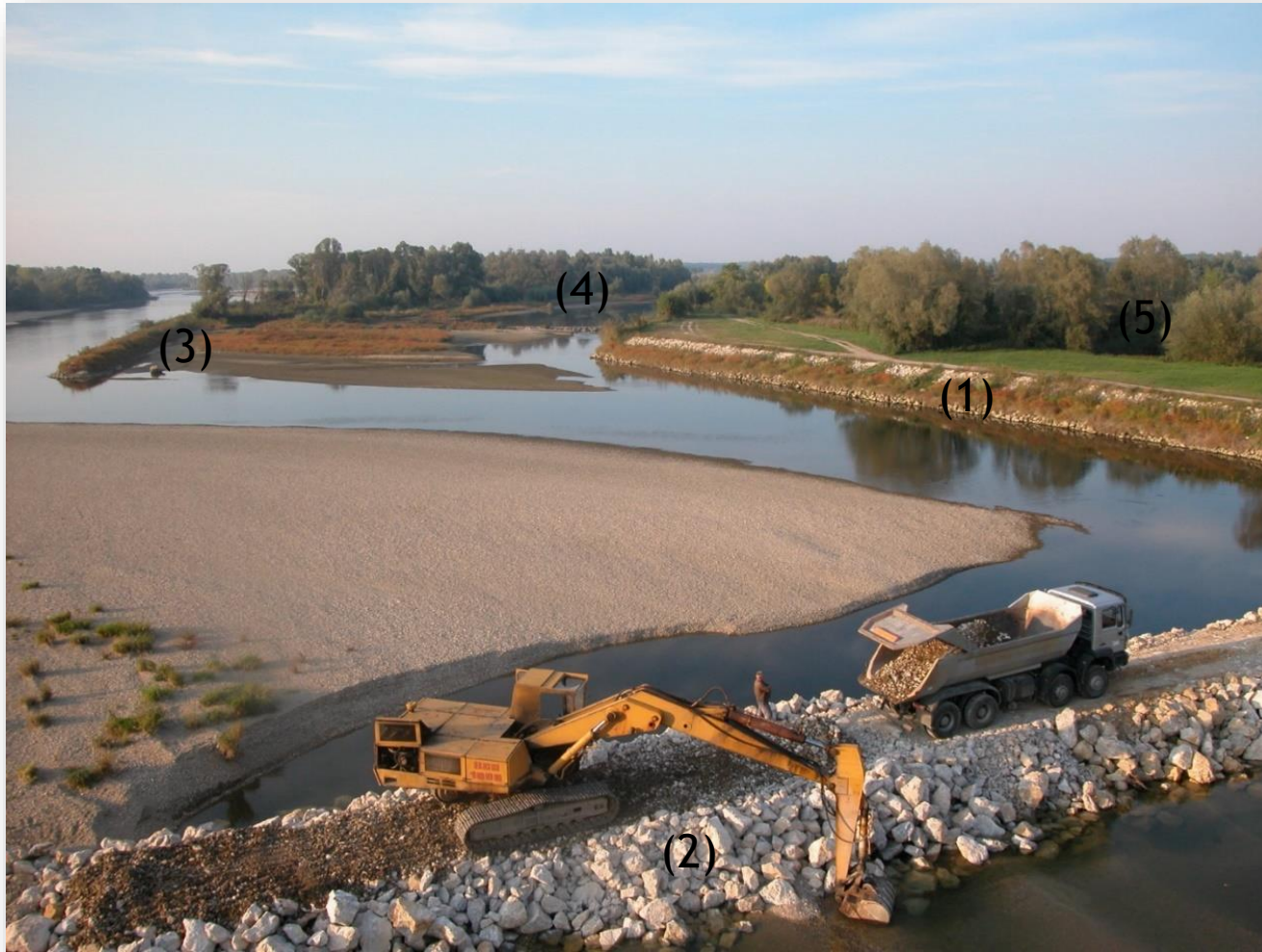
Bank reinforcements (1), groynes (2, 3), transversal fills (4) and flood dyke (5) at Drava to protect infrastructure such as bridges and settlements (Arno Mohl).
