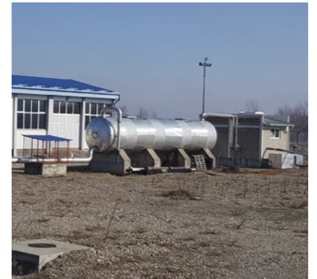
The production well (GD-2), the buffer tank and the building of the heating station
