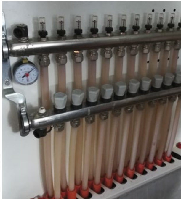
The heating system in the waterpark (photo by I. Bobovečki)
