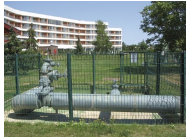
Several hotels, indoor and outdoor swimming pools are heated with geothermal energy at Terme 3000
