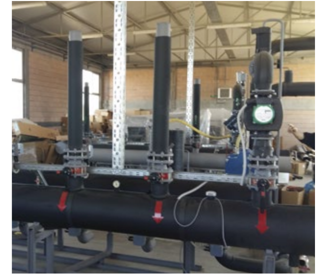
The modern heating plant
