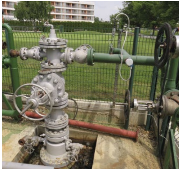
The monitoring system at the wellhead of one of the wells.
