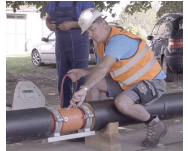
Construction work of the geothermal heating system. Mr. Christian Mrazek, Head of Business Team, Rehau SEE.
