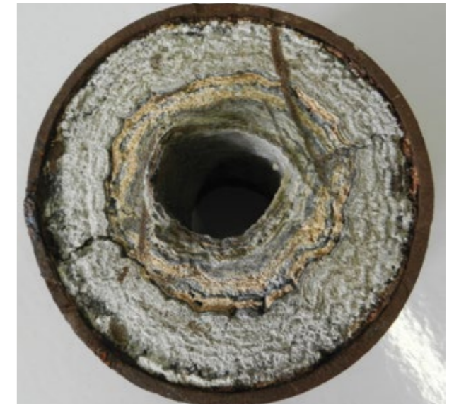
Carbonate scaling from thermomineral water at Terme 3000 (the diameter of the pipe is 16 cm)
