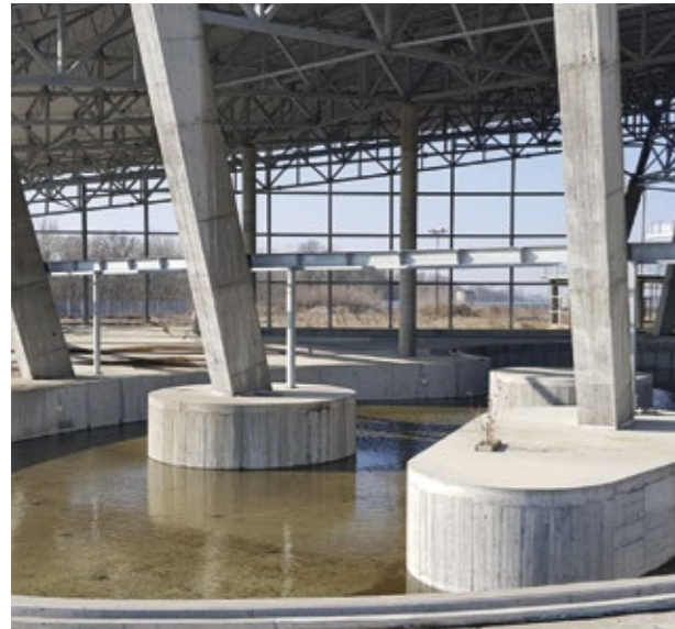
Current status of the first stage facilities of the aqua park construction, February 2019
