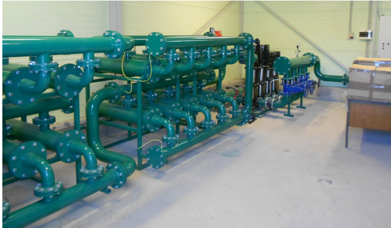
Filtering system prior to reinjection, Lendava, Slovenia
