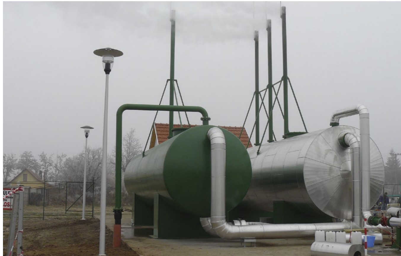
Production well and degassing buffer tank at the Makó cascaded system, Hungary
