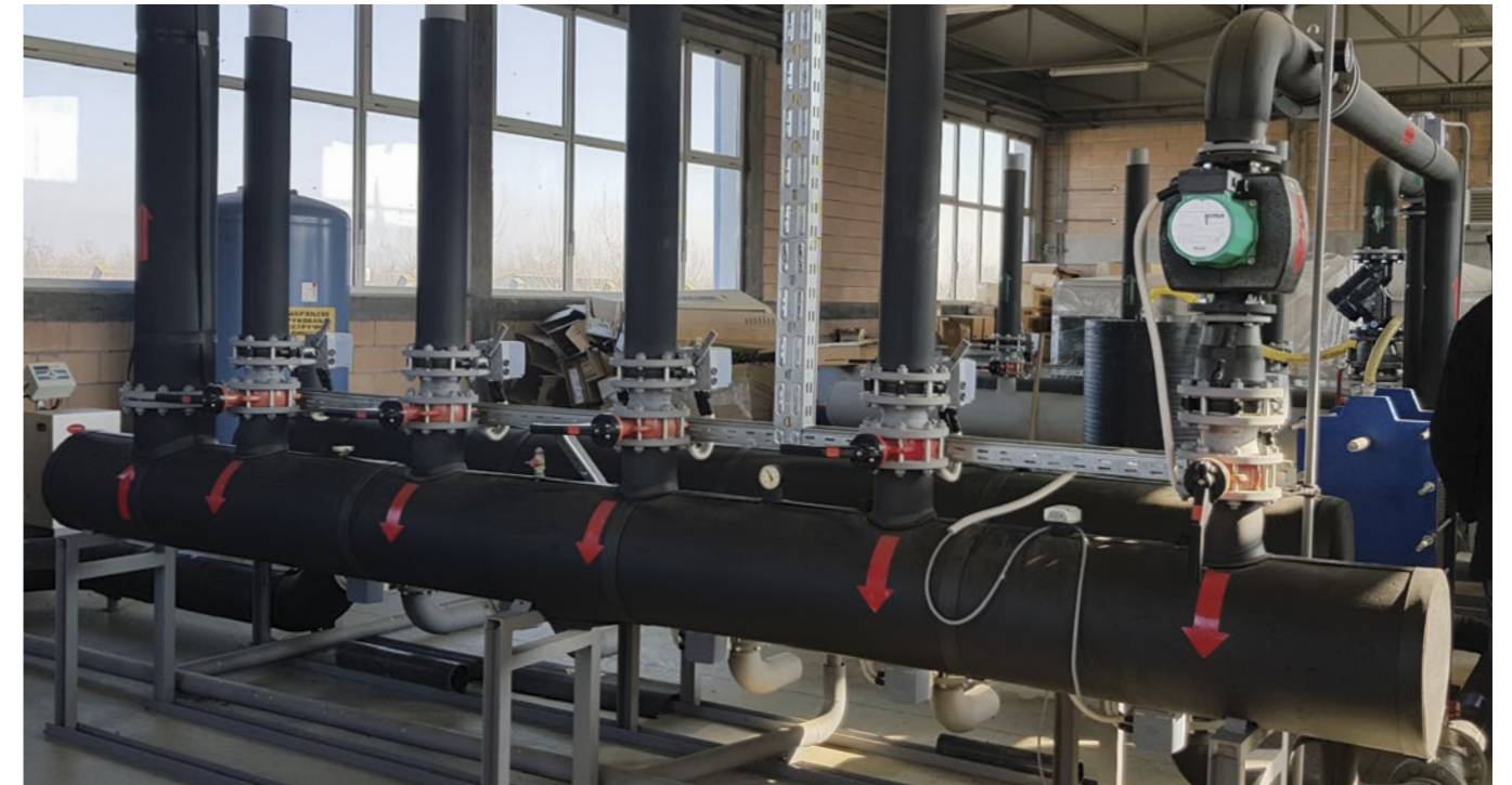
Heating station at Slobomir, Republic of Srpska, Bosnia and Herzegovina
