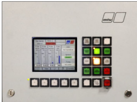
Local Operator Panel (LOP)
