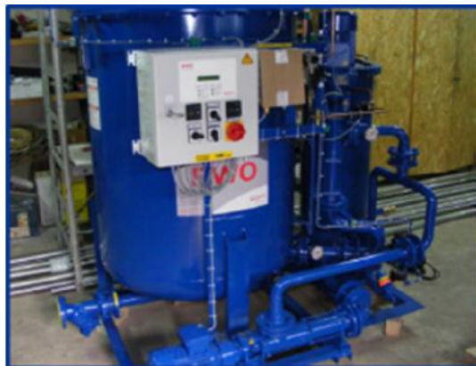
Figure 73: Equipment used for the compact wastewater treatment plant (Giurgiu)
