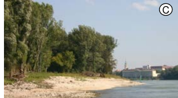
River Bank Restoration - removal of 1,2 km stone amour along the river bank
