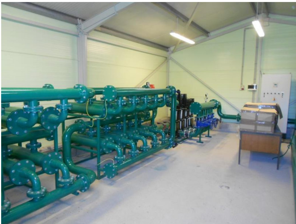
Figure 30: Fibre filters for waste thermal water before being reinjected into Le-3g well in Lendava geothermal district heating system, Slovenia
