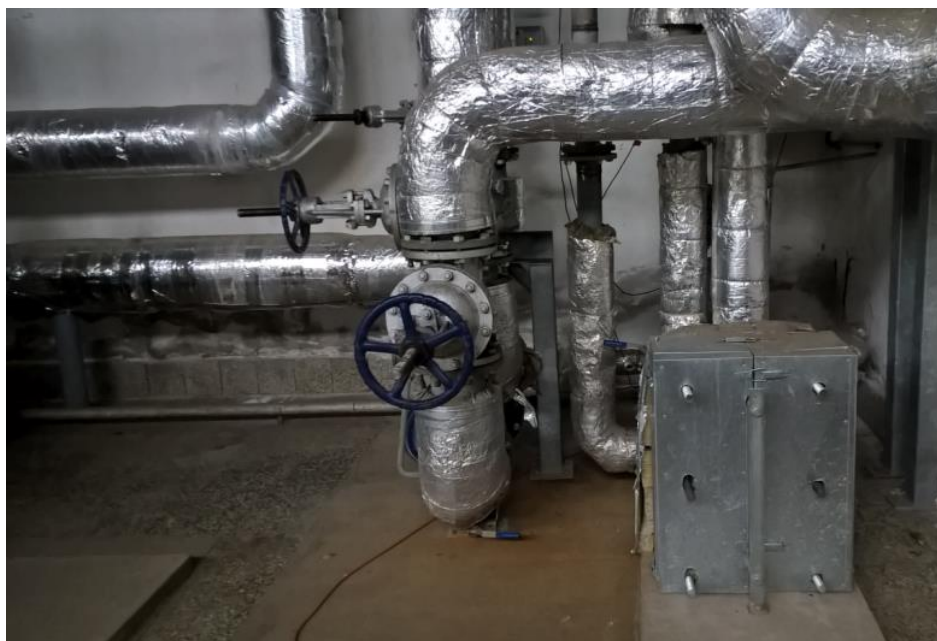
Figure 28: The heat exchanger with mechanical equipment in the Szentlőrinc geothermal district heating system, Hungary
