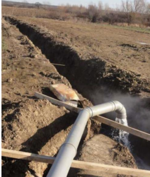
Figure 29: Discharge of cooled geothermal water (30 °C) into a melioration channel in Bošnjaci (Croatia) where the thermal water is used for heating of greenhouses
