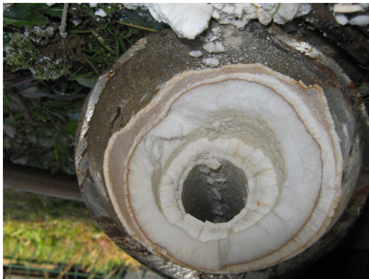
Figure 32: High mineralization and CO 2 degassing of the water cause scaling which clogs the well (Benedikt, Slovenia)
